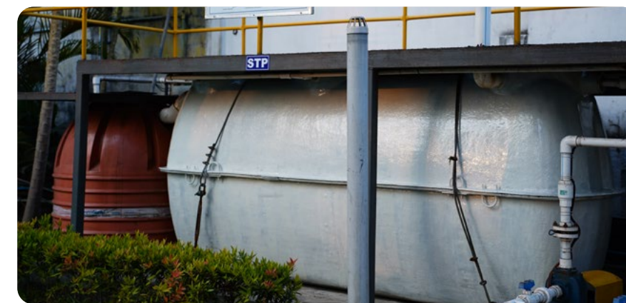
Sewage Treatment Plant in Samali, West Bengal, India
